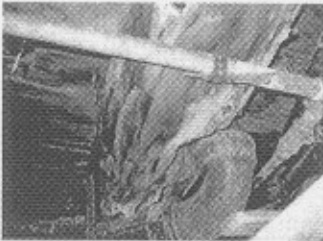
Photo 10 – Cut & Deteriorated Floor Beam – Boiler Room
