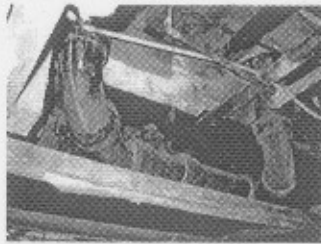
Photo 11 – Notched Joists – Boiler Room
