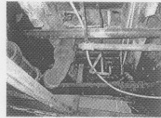
Photo 12 – Notched Joists - Boiler Room
