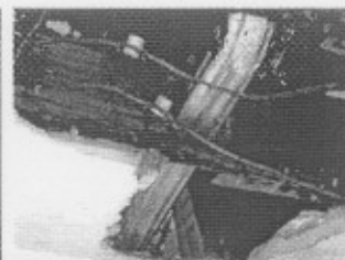
Photo 19 – Roof Drain through Roof Joist
