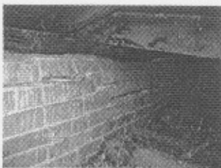
Photo 26 – Failed Masonry Support Wall
