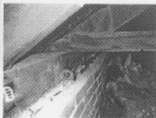
Photo 27 – Failed Masonry Support Wall
