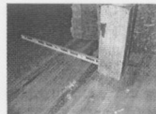
Photo 34 – Dining Room Column Settlement
