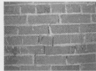
Photo 32 – Cracked Brick Gable
