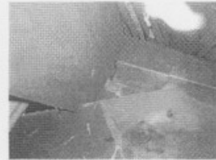
Photo 30 – Failed/Cracked Roof Members
