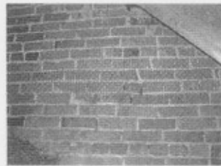
Photo 31 – Cracked Brick Gable
