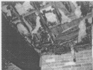
Photo 37 – Rotted Roof Timber (1957)
