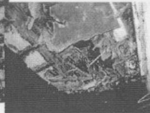
Photo 39 – Rotted Roof Timber (1957)
